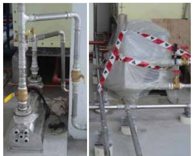
Pipes connection from Booster Pump
