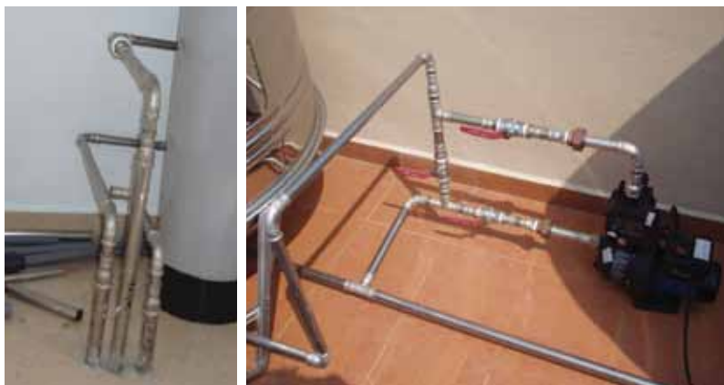
Pipes Connection at Water filter tank
