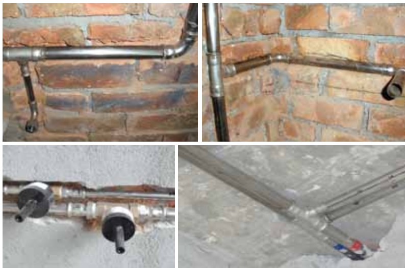
Internal Plumbing (Hot and Cold Water)
