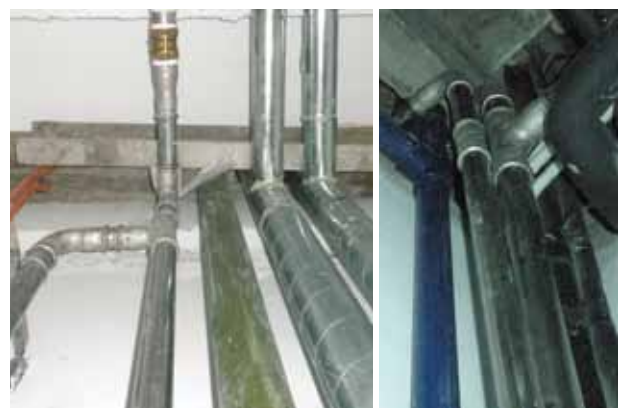
Riser Pipes for High Building
